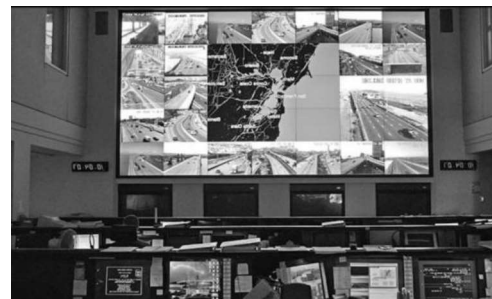
Figure 5. Traffic management center
